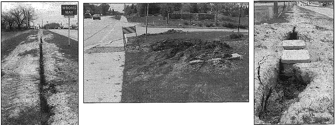
Figure 3: Examples of Improper R/W Restoration
